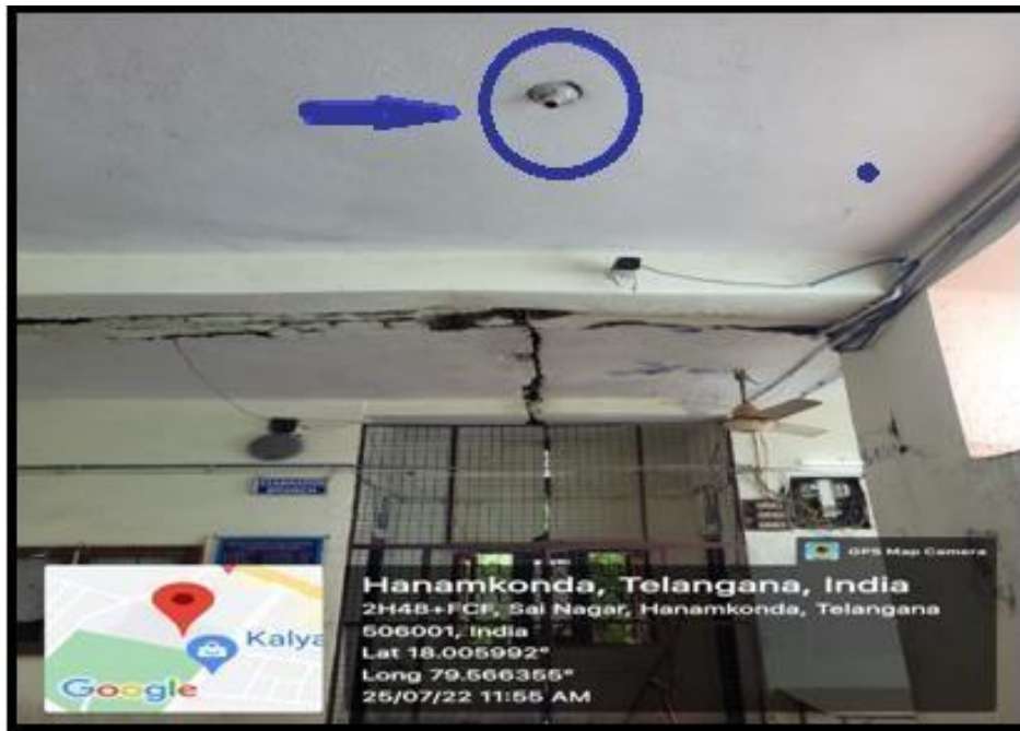
CC Camera in front of the Examination Branch
